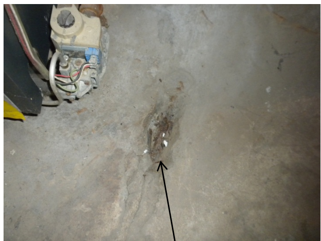
E3. Disconnected oil pipe
