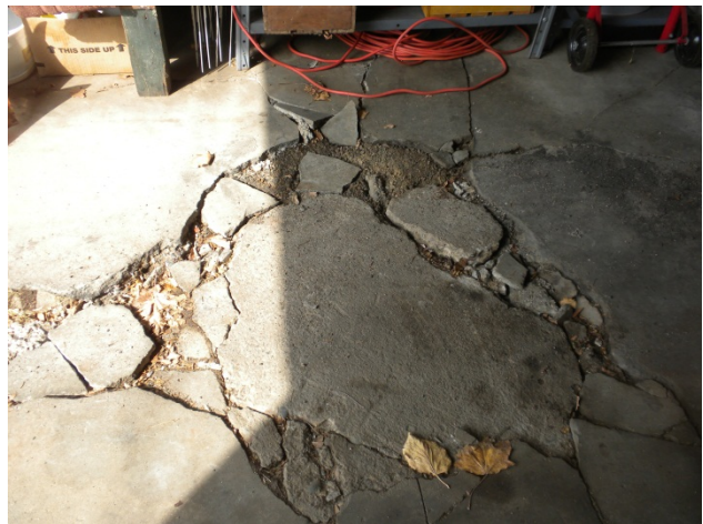
B3. Cracked garage floor
