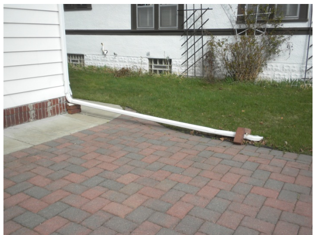
A2. Over extended downspout extension
