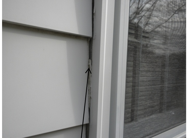
B1. Cracked & missing caulking
