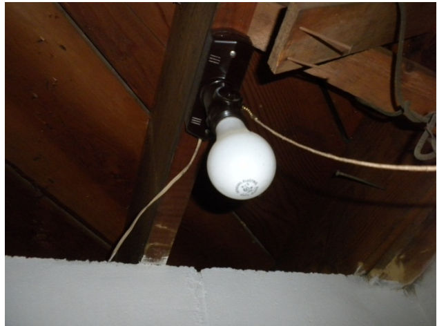
D2. Extension cord fixture wiring
