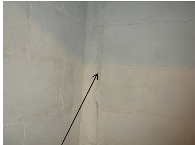
C1. Vertical shear cracks / bowed wall
