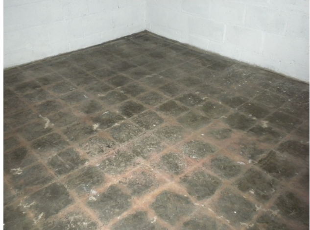
C1. Missing tiles / glue remains
