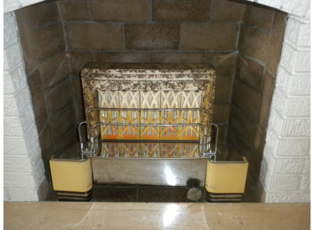
G3. Unsafe gas heater
