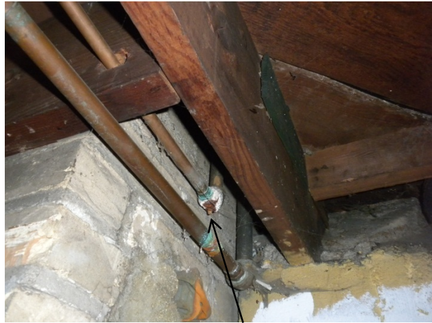
E1. Corroded connection
