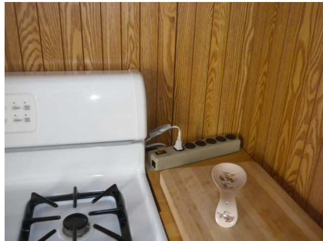
G1. Extension cord kitchen outlet
