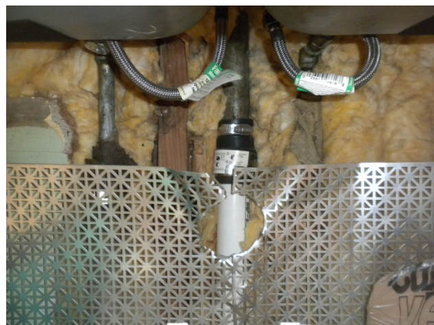
G1. Water pipes in unheated space / improper connector
