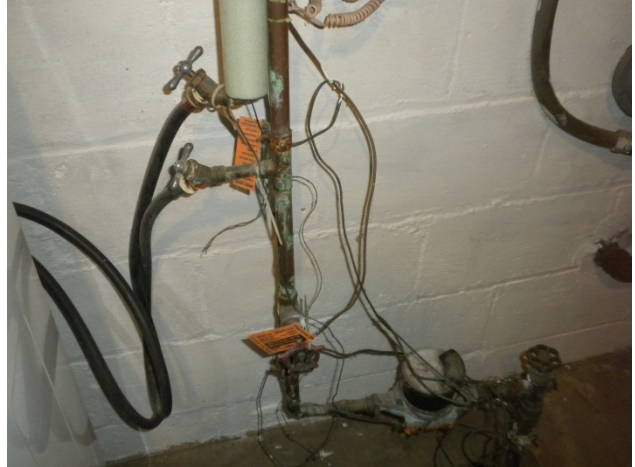
E1. Improperly located clothes washer faucets
