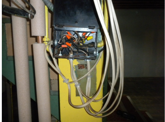
D2. Unsealed panel & unprotected wiring
