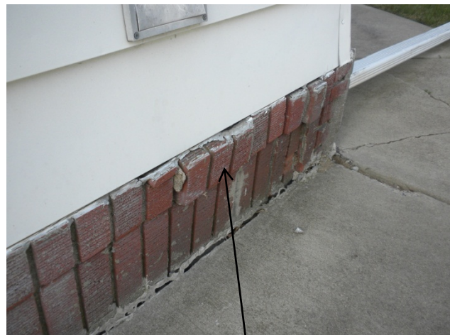
B1. Loose & tipped bricks
