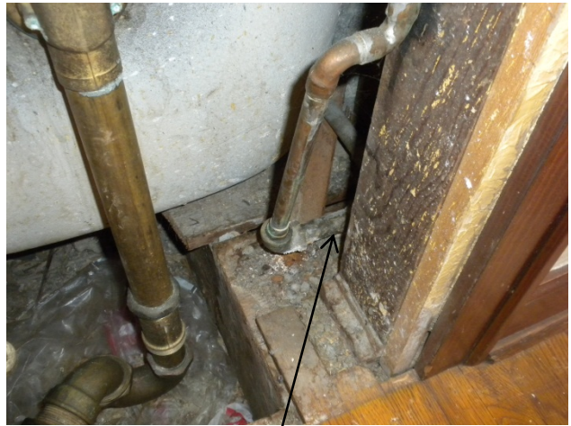
G3. Iron vertical water pipes
