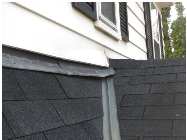
B2. Loose wall flashing
