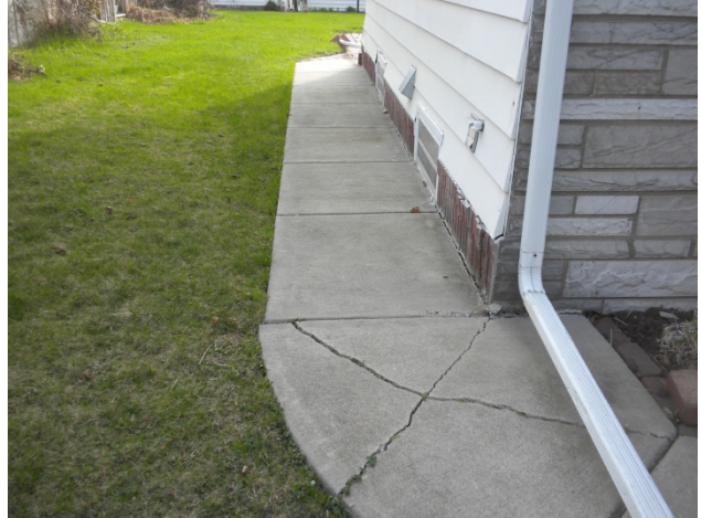
A2. Flat & cracked sidewalk
