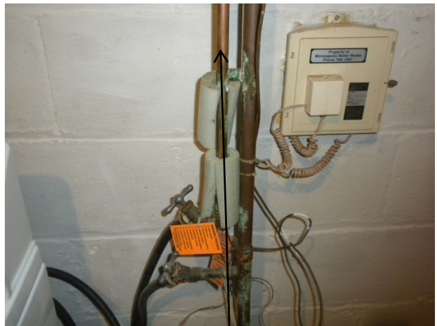
E1. Undersized water pipe
