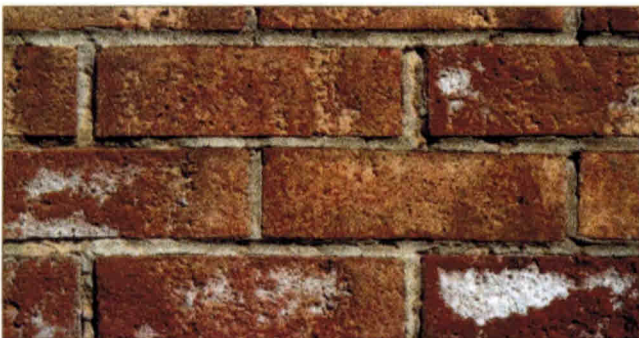
Photo 3, Efflorescence in limited areas
