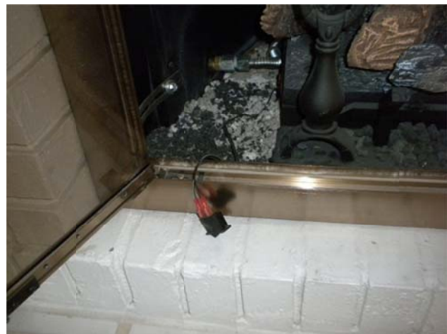
3. Unprotected fireplace wiring
