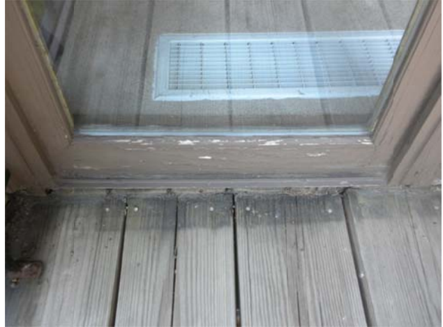
7 & 8. Worn patio doors
