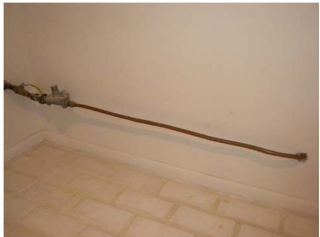
9. Unprotected closet gas pipe
