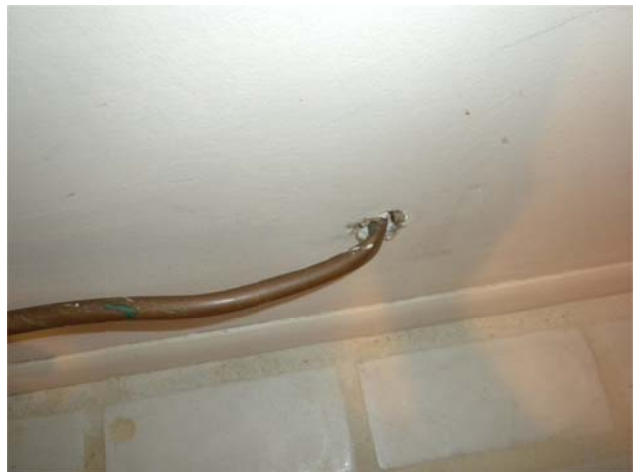
9. Kinked fireplace gas pipe
