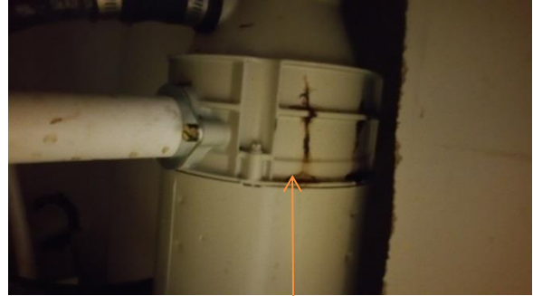
Cracked & leaking disposal
